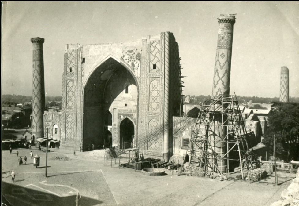
Mosque under construction, ca. 1900 Photograph by S.M. Dudin Courtesy of Andrew Hale Anahita Gallery, Santa Fe, NM
